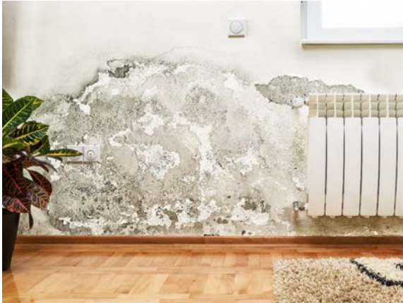
Damp - Mould - Condensation
